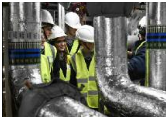
CLOSER LOOK: Students have a detailed tour of the energy centre.
